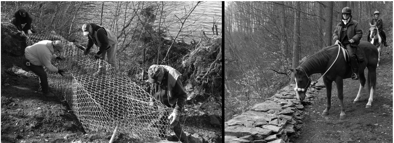
Left: Volunteers ready a series of gabions to be filled with rocks to make a Nockamixon State Park trail usable once again. Right: Riders check out the finished trail work.
